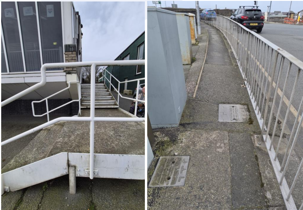
Figure 19: Examples of access barriers identified during community mapping in North Wales, including stepped access to a GP surgery and a narrow pavement restricted by railings and communication boxes.
