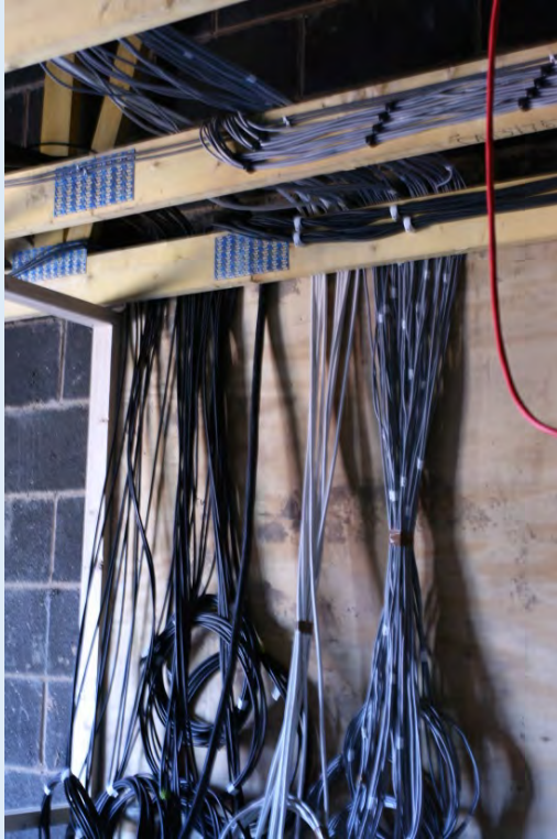
Pre-installed Adaptive Technology infrastructure
