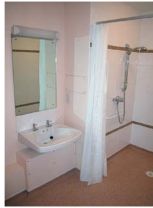
Ensuite showing flush floor shower and knee space below wash hand basin
